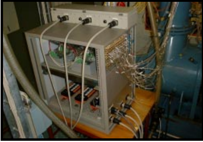
Fig. 8 The measurement system installed in the casing
